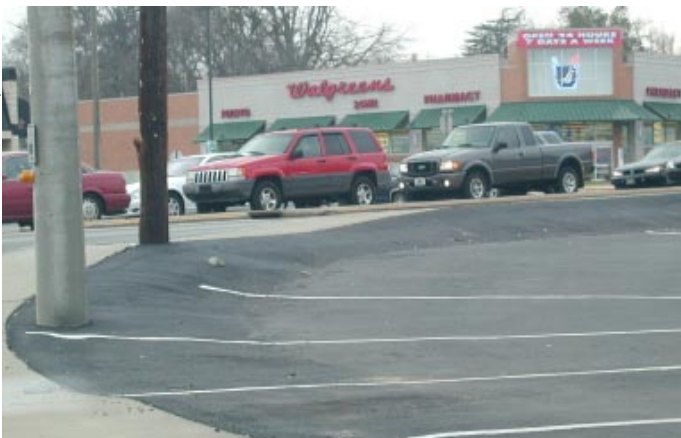
Greenville, SC: Parking lots and streets are one of the largest sources of impervious cover.
