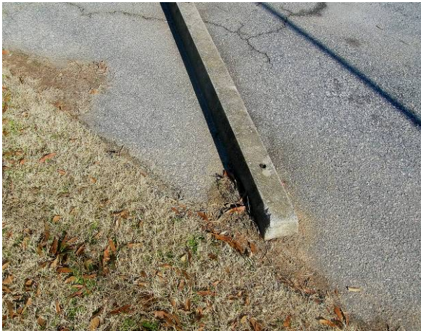
Parking area landscaping with no curbing allows for more effective infiltration of storm water when it is at grade or below (Laurens, SC). Source: Upstate Forever
