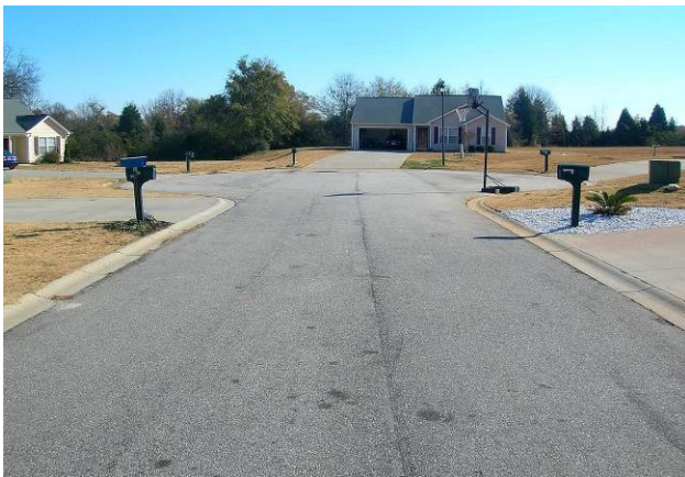
On this cul-de-sac street, pavement could easily be narrowed by 4 to 6 feet (Gray Court, SC). Source: Upstate Forever
