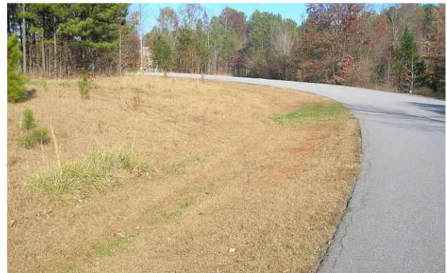
The gentle slope of the swale on the side of this street is an easily maintained area that can be mowed (Laurens County, SC). Source: Upstate Forever
