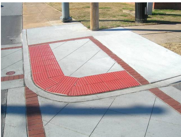
Small radius curb with mountable curbing. Note tire tracks across the ramp apron (Clinton, SC). Source: Upstate Forever
