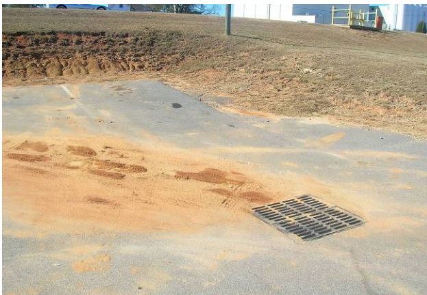
Grading that slopes away from landscaped areas provides little opportunity for natural infiltration of stormwater (Gray Court, SC). Source: Upstate Forever
