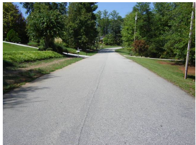
An example of a narrow street with no curb and gutter (Oconee County, SC). Source: Upstate Forever
