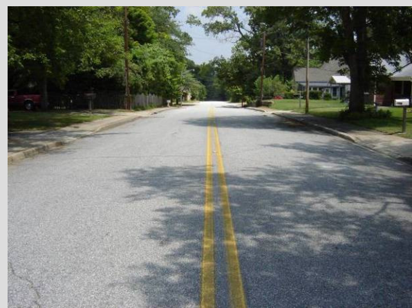
An example of a street that is approximately 40 feet wide. The amount of unused pavement represents a missed cost savings opportunity for the developer of at least 8 to 10 feet (Westminster, SC). Source: Upstate Forever
