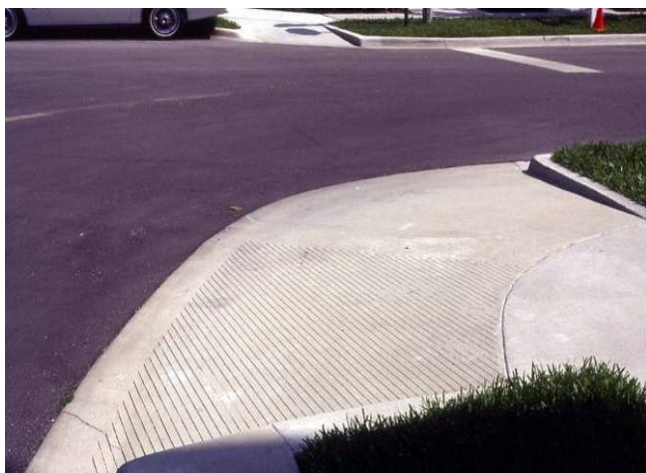
Small radius curb with mountable curbing on a residential street. Note tire tracks across the ramp apron (Celebration, FL). Source: The Lawrence Group
