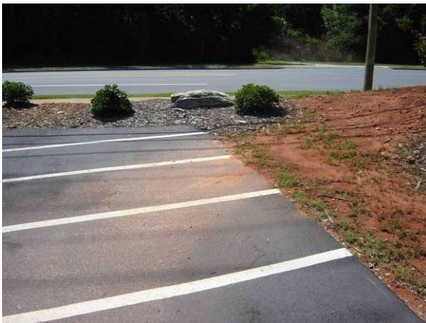
Grading that slopes away from landscaped areas provides little opportunity for natural infiltration of stormwater (Salem, SC). Source: Upstate Forever
