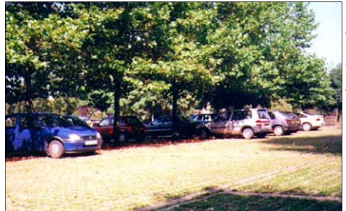
A parking lot with Grasscrete™ interlocking pavers. Bordered by a stream and with no option for piped drainage, this parking lot has been draining naturally for 20 years (location unknown).
