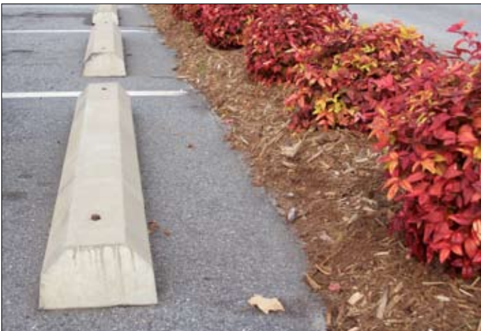
Parking area landscaping with no curbing would allow for more effective infiltration of stormwater if it were at grade or below (Anderson County, SC).
