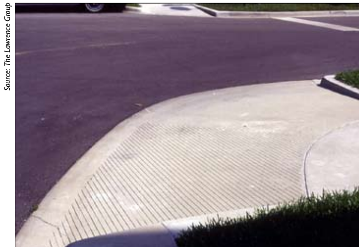
Small radii with mountable curbing on a residential street. Note tire tracks across the ramp apron (Celebration, FL).
