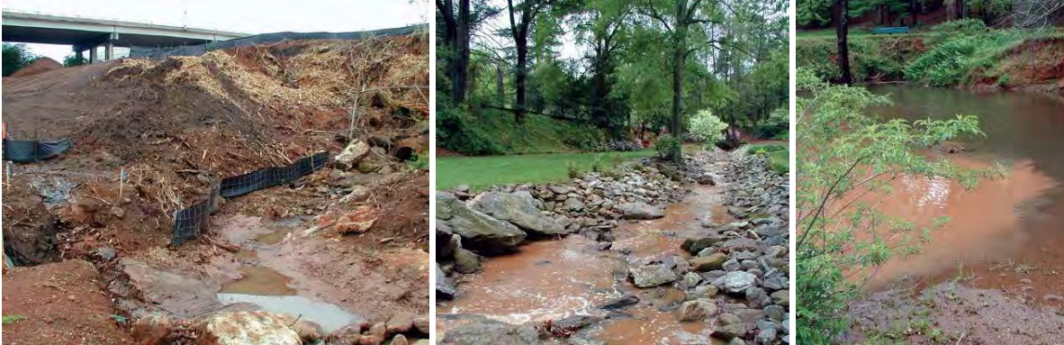
This development site in Greenville is typical of many in the region, with extensive bare dirt and failing erosion control structures. It took only a 20-minute shower to send a plume of sediment down to the nearest stream and into the Reedy River.
